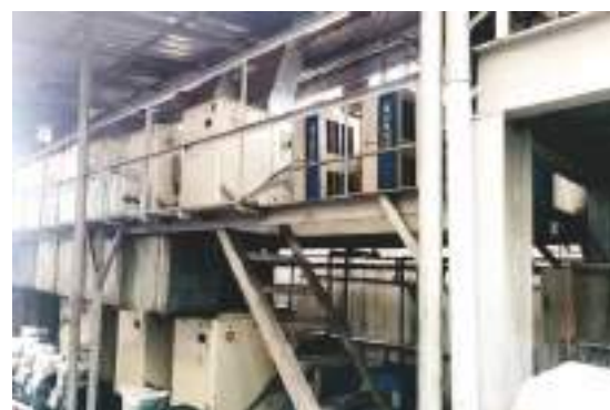
>> Air Compressor Placed Outside Workshop
