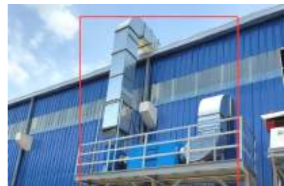
>> Exhaust Gas Treatment System
