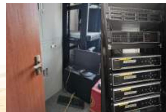
&gt;&gt; Server Room
