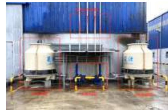
>> Cooling Water System
